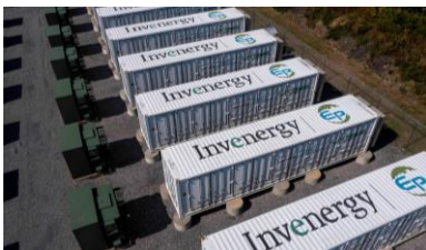
Storage at Invenery's Beech Ridge Energy Center in Greenbriar County, West Virginia
